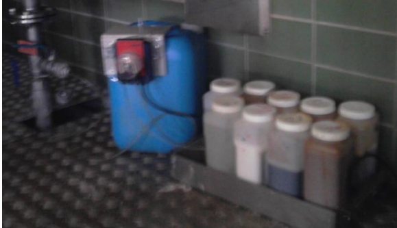
Photo 1 Dosing station for EWT 21 (25 L plastic container and Jesco hose pump)
